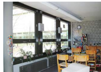
Markt Indersdorf primary and secondary school: installation of centrally-controlled M-WRG units in the course of renovation
